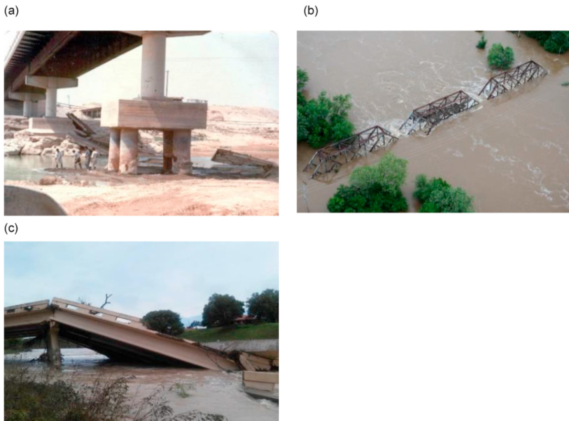
Figure 4. Bridge failures due to hydraulic. (a) Foundation scouring. (b) Bridges submerged by flood. (c) Bridge collapse due to flood
