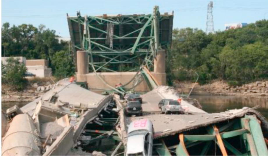
Figure 1. Bridge failures due to design errors (Defects in design theory)
